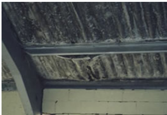
Damaged asbestos cement roof
