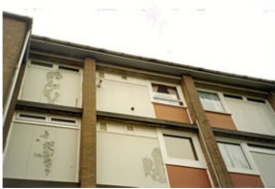
Damaged asbestos panelling
