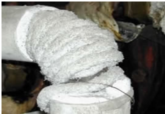
Pipe insulated using both asbestos lagging and rope
