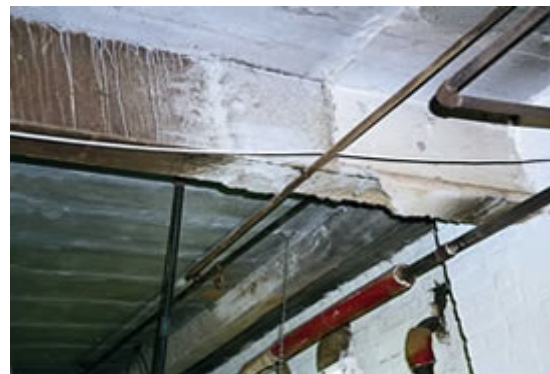
Sprayed 'limpet' asbestos coating which has been partly removed
