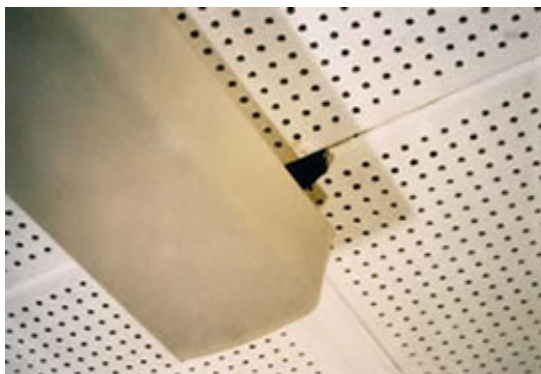
Perforated AIB ceiling tiles damaged around the light fitting
