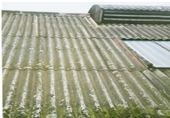
Asbestos cement roof (weathered exterior)
