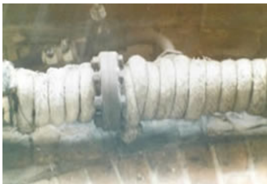
Asbestos rope used as insulation on a pipe
