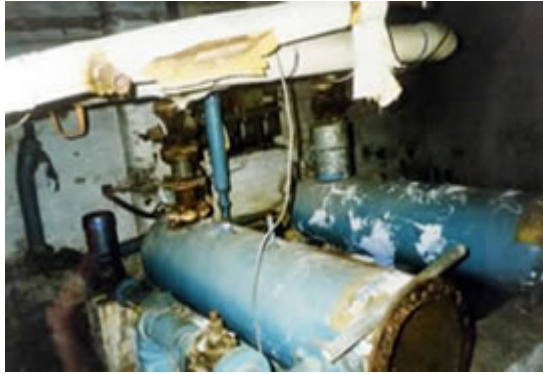
Damaged asbestos pipe lagging and debris
