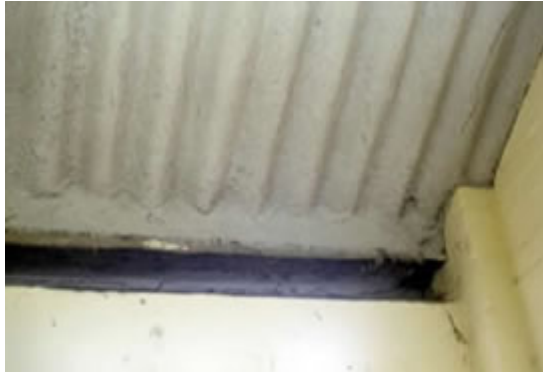
Sprayed 'limpet' asbestos on the underside of an asbestos cement roof
