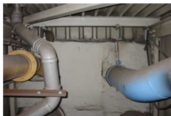
Wall with trowelled loose asbestos
