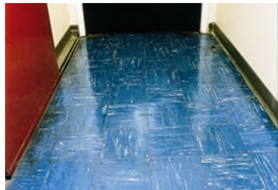
Asbestos containing vinyl floor tiles
